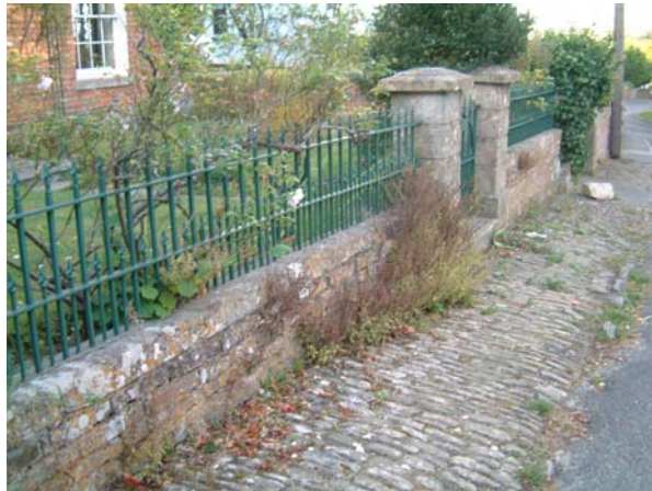
No.2 Church Road of 1840, stone copings and gate piers, iron railings and pitched limestone
